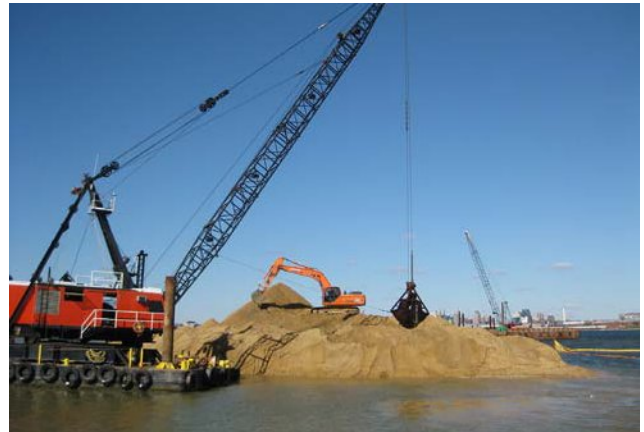
In 2007, the Maryland Port Administration began construction of the containment dikes for the Masonville Dredged Material Containment Facility. (photo: Kaitlin McCormick)
